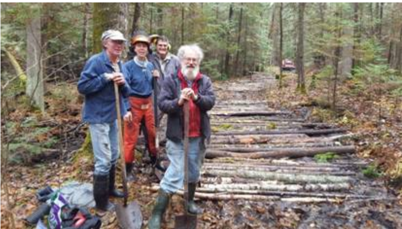
Cutting and laying corduroy (and digging drainage trenches) on muddy sections of R loop
