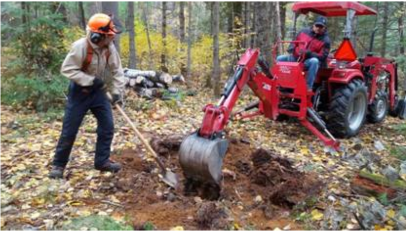
Digging stumps out of the new R loop “re-route” trail (next to Balmer Bay Road)
